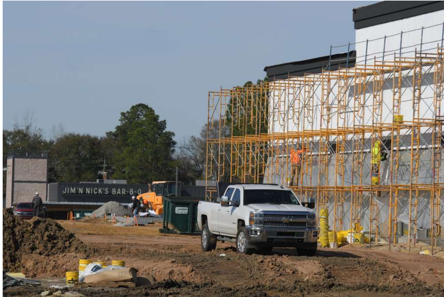
Commercial construction on Highway 80 near Harbor Freight and Lowe's on Wednesday, Dec. 13. Credit: Scott Bryant, Statesboro Herald.
