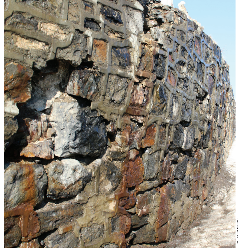
REPLACEMENT NEEDED: A falling apart High Street retaining wall needs to be rebuilt.
