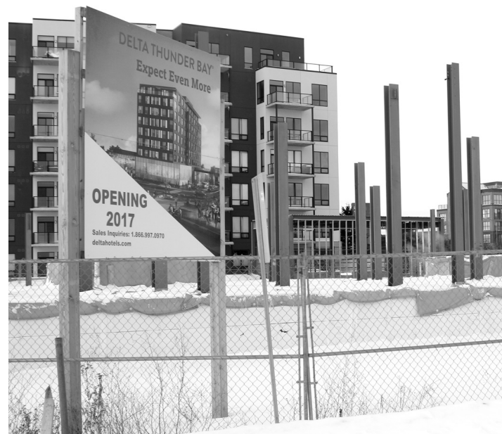
OPENING SOON?: Delta's waterfront hotel has been in the works for several years.
