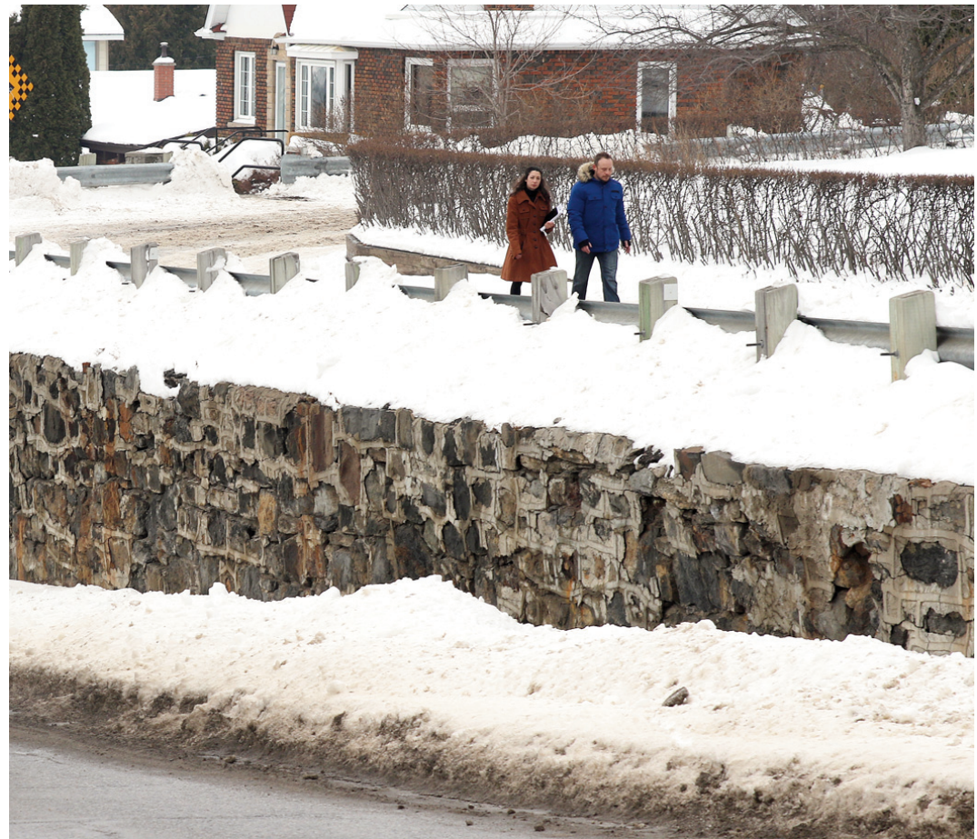
THE ART OF WAR: The future replacement for this crumbling High Street retaining wall is under consideration.
