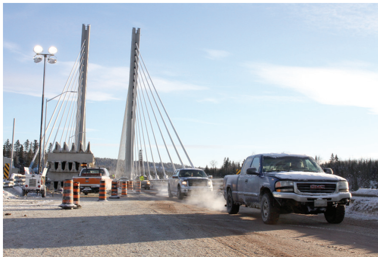
BROKEN BRIDGE: The Nipigon River Bridge was closed for 17 hours in January.
