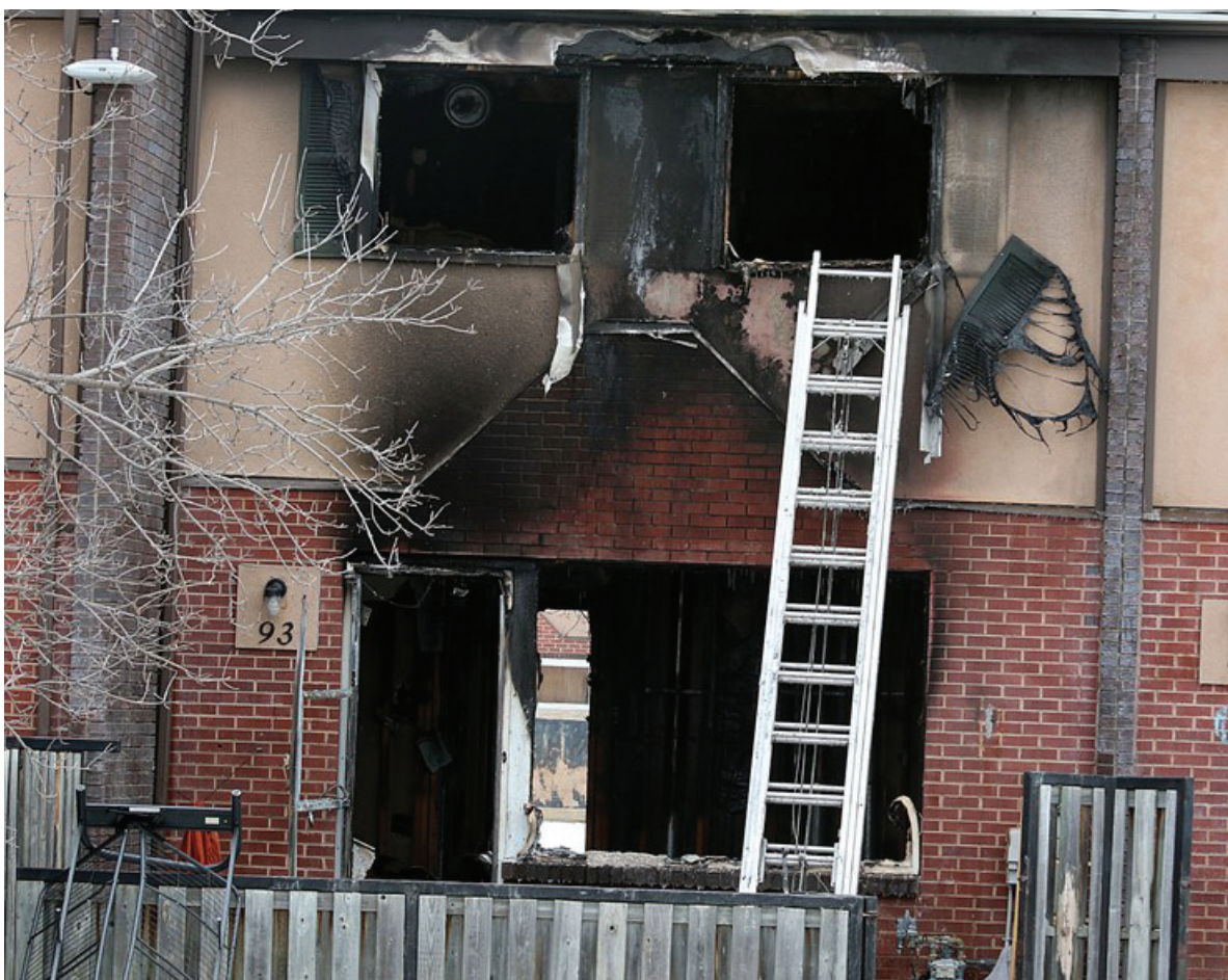
HEAVY DAMAGE: No one was hurt when fire swept through this Limbrick Street residence on Saturday morning, gutting the home in the process.
