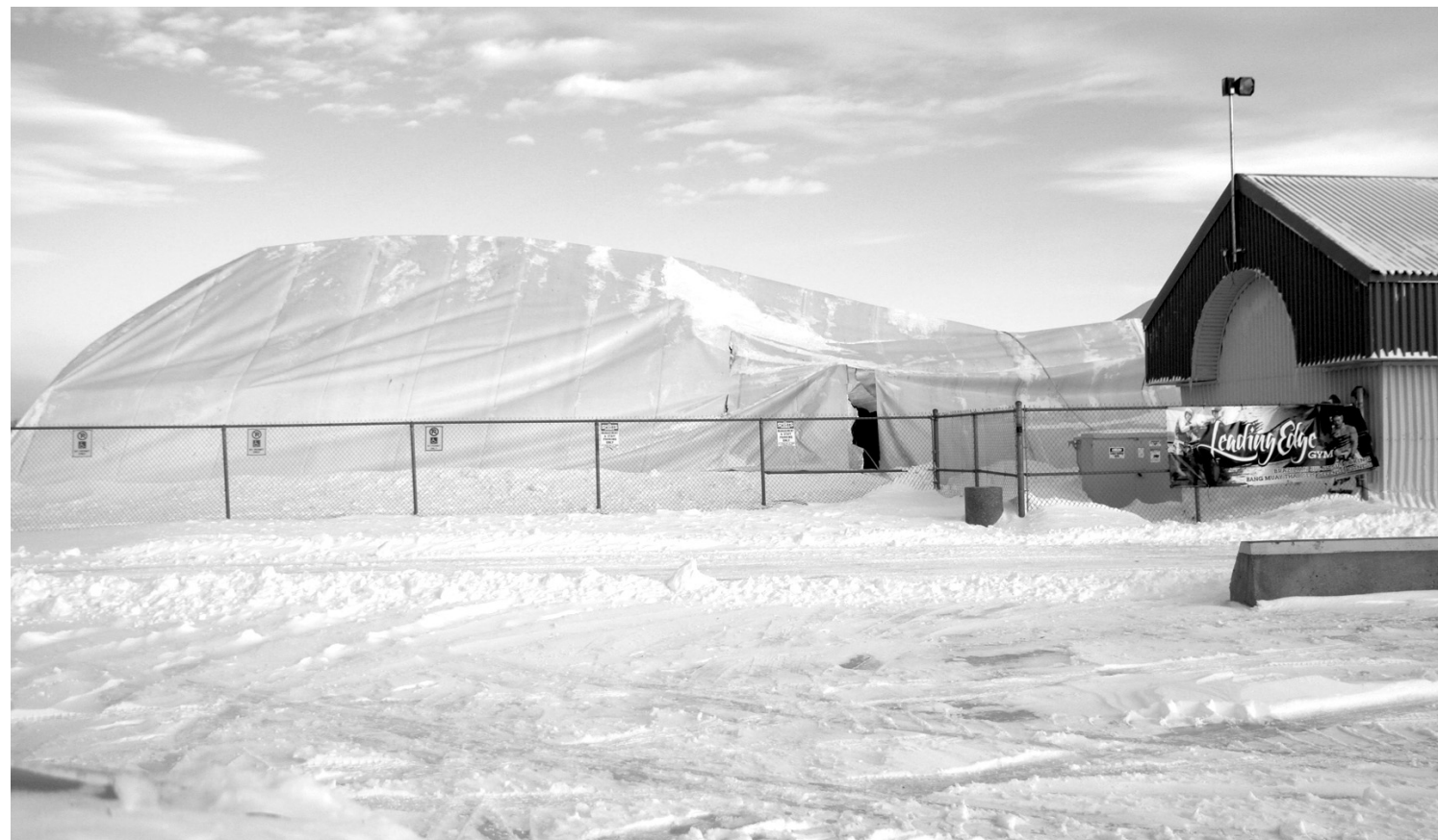
RIPPED OPEN: Last Friday's snow storm tore a gash in the bubble at the Sports Dome. The damage is expected to keep the facility closed for up to a month.
