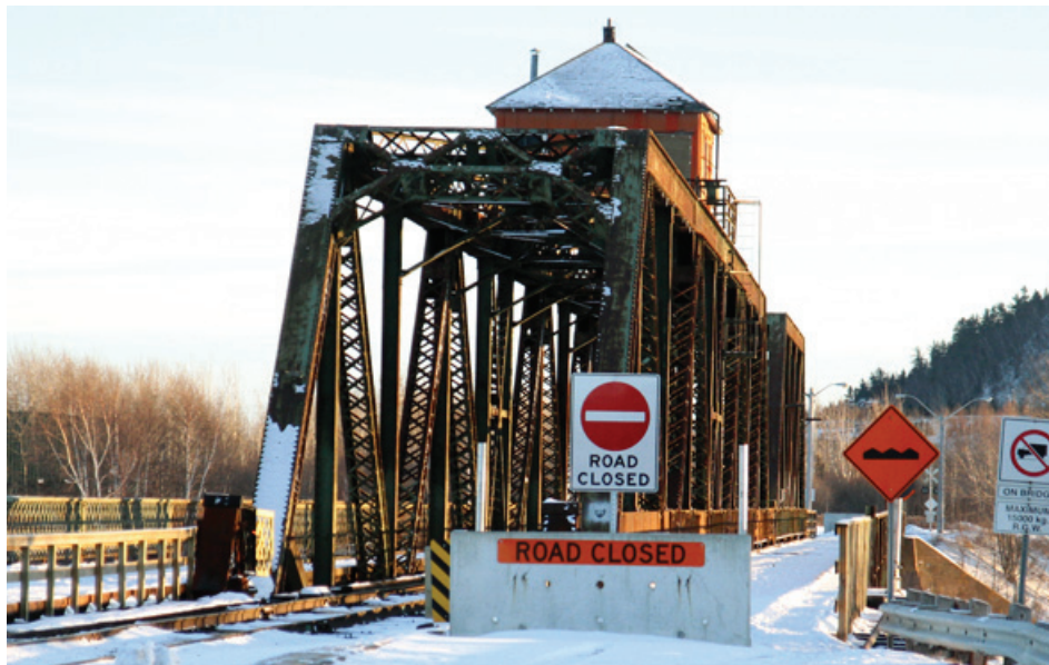
STILL SHUT DOWN: The James Street Swing Bridge has been closed to vehicles since October 2013.
