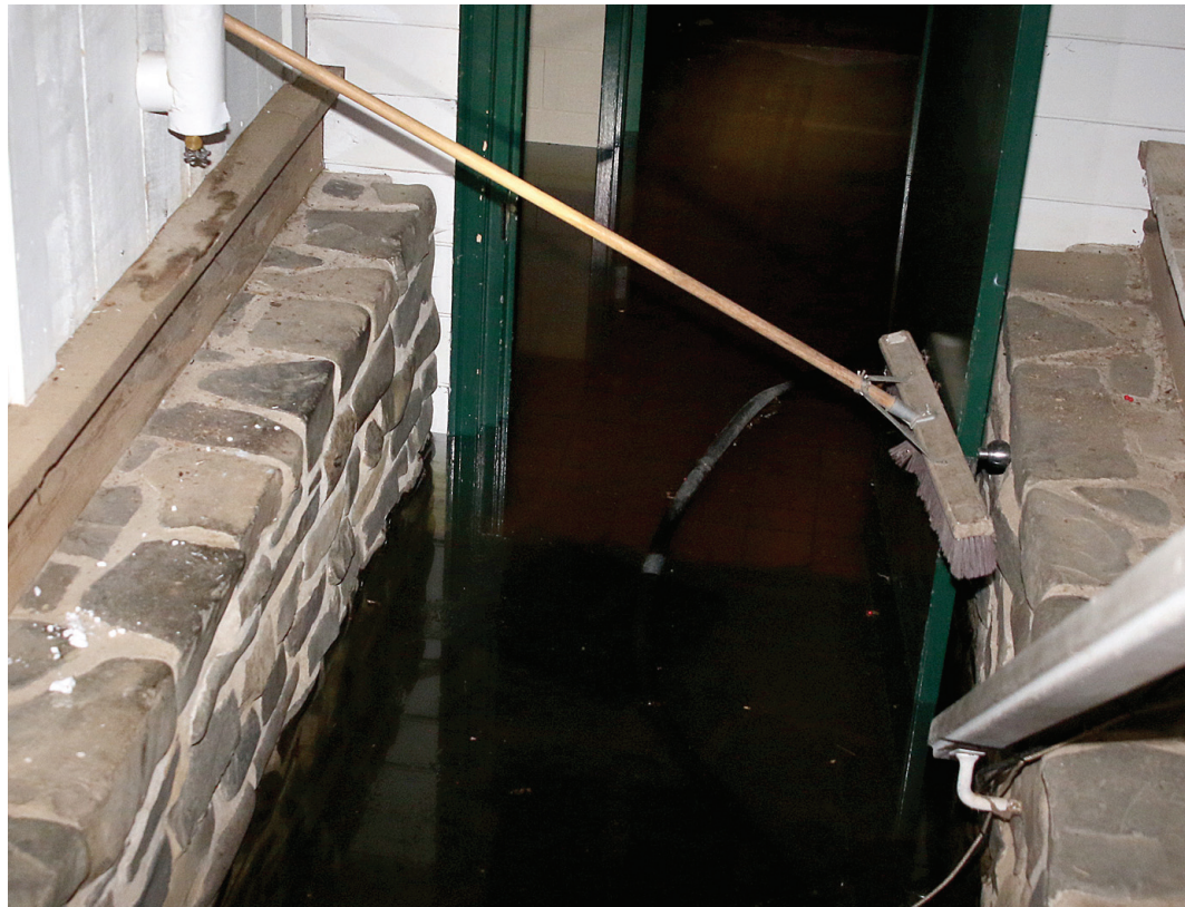
UNDER WATER: Flooding of the Great Hall at Fort William Historical Park has left the basement submerged.
