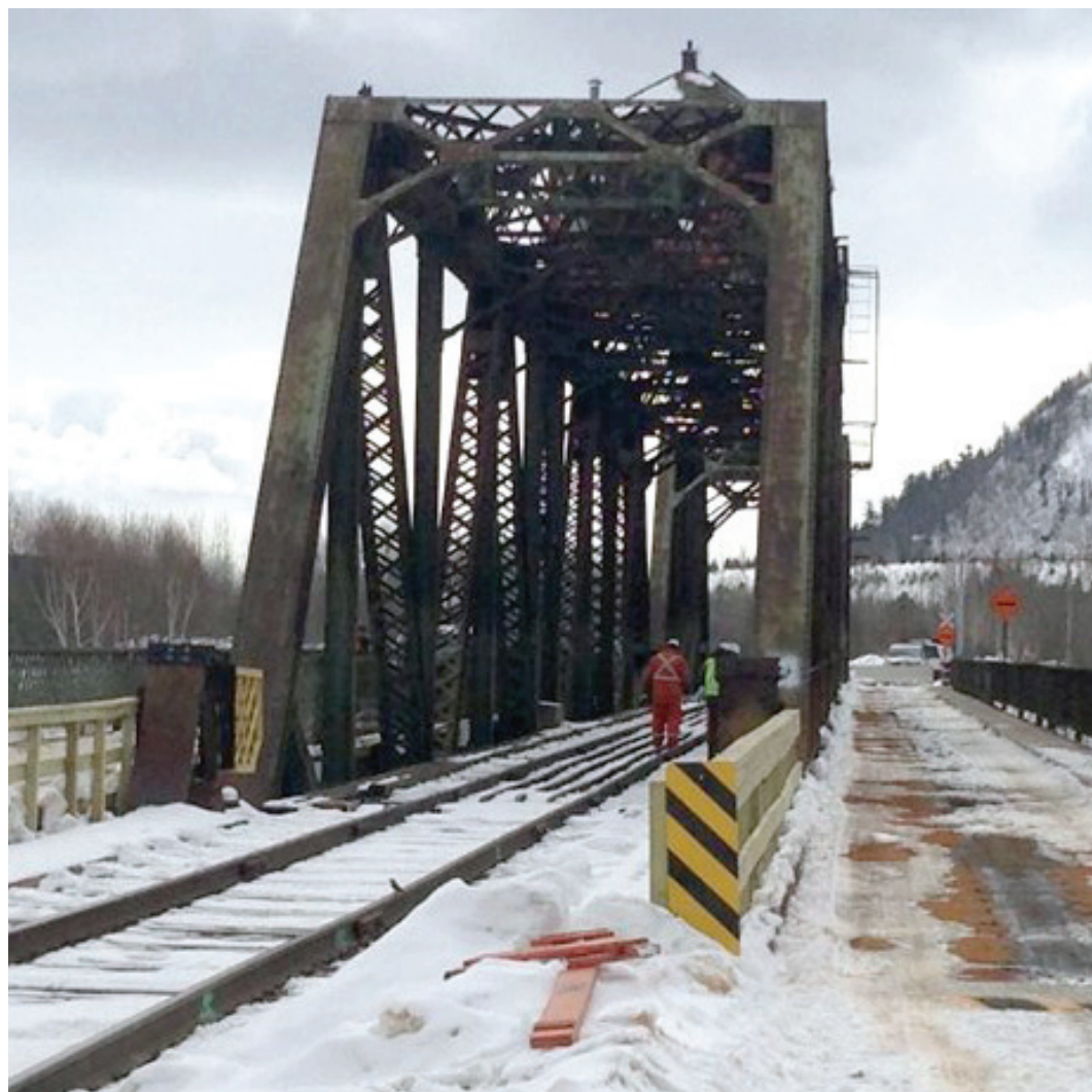
SPIC AND SPAN: Workers inspect the James Street Swing Bridge, which closed in October 2013 after a massive fire.
