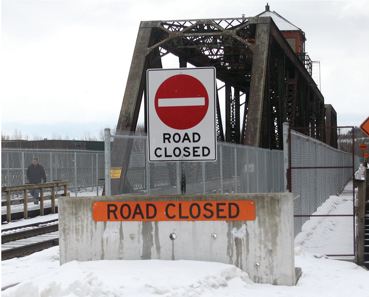
FINALLY OVER: Barring a setback, the James Street Swing Bridge should open to vehicular traffic again at some point in 2019.
