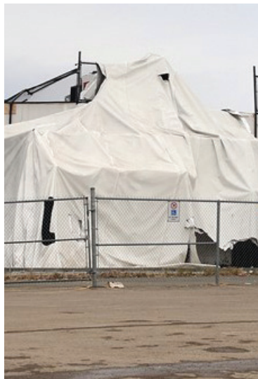
MESS LEFT BEHIND: The Sportsdome collapsed in November 2016.
