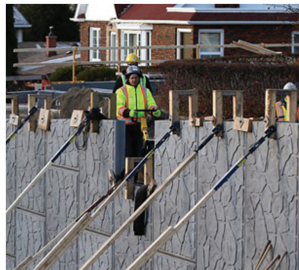
MORE TO DO: A worker completes work on the retaining wall last fall.
