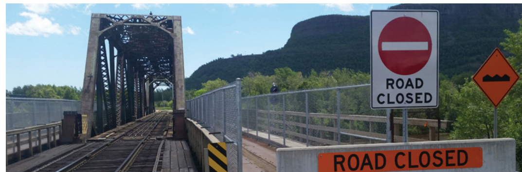
SET TO REOPEN: The James Street Swing Bridge has been closed since a fire broke out in October 2013.
