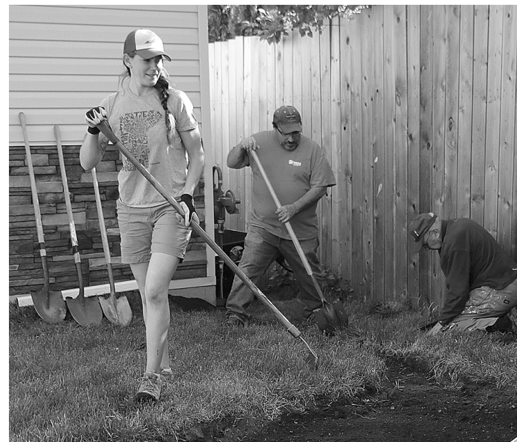
INTO YOUR GARDEN: Eco-Superior's Julia Prinselaar helps build a rain garden at a Dease Street home built last year by Dion Horton (centre) and Habitat for Humanity.
