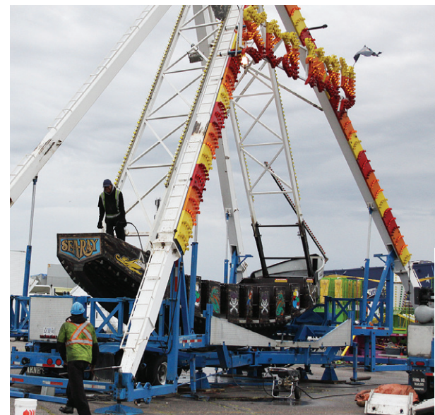
READY TO GO: Crews work to set up the Sea Ray ride on the CLE grounds last Friday.
