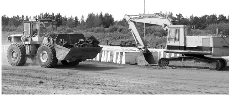
WORK UNDERWAY: Work continues at the Thunder Valley Development Race site, which will be the future home of the Dairy Queen International Speedway.
