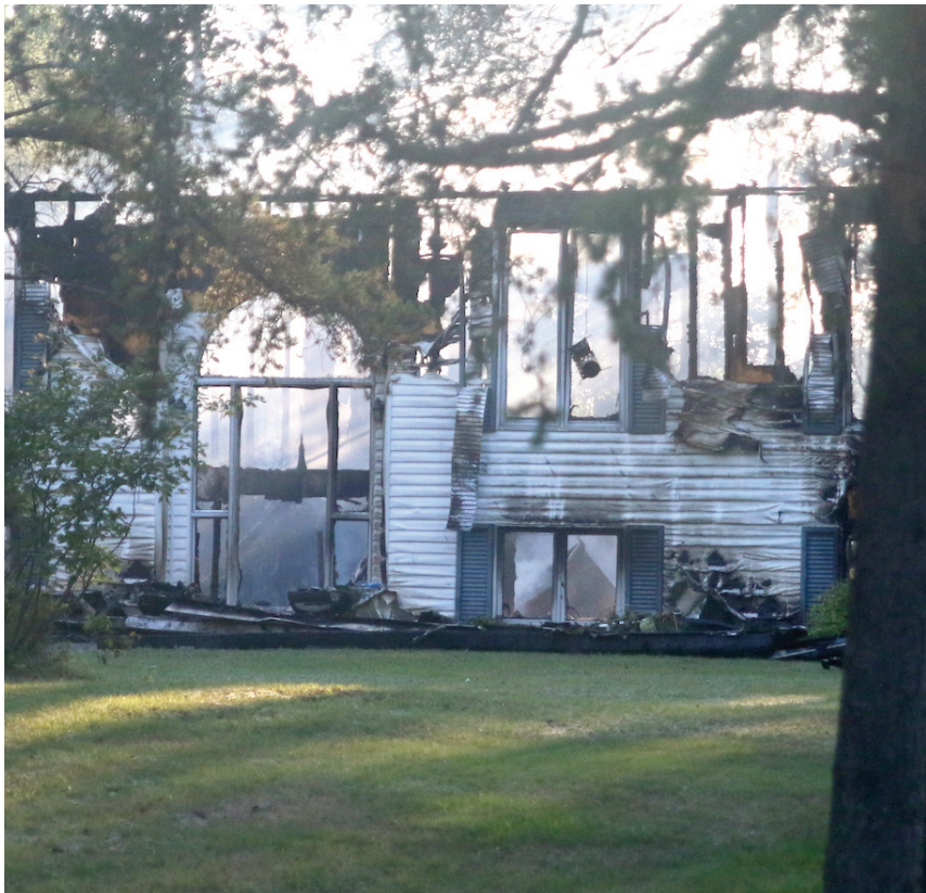
AFTERNOON FIRE: The remains of a Pennock Drive home destroyed in a Sunday blaze.
