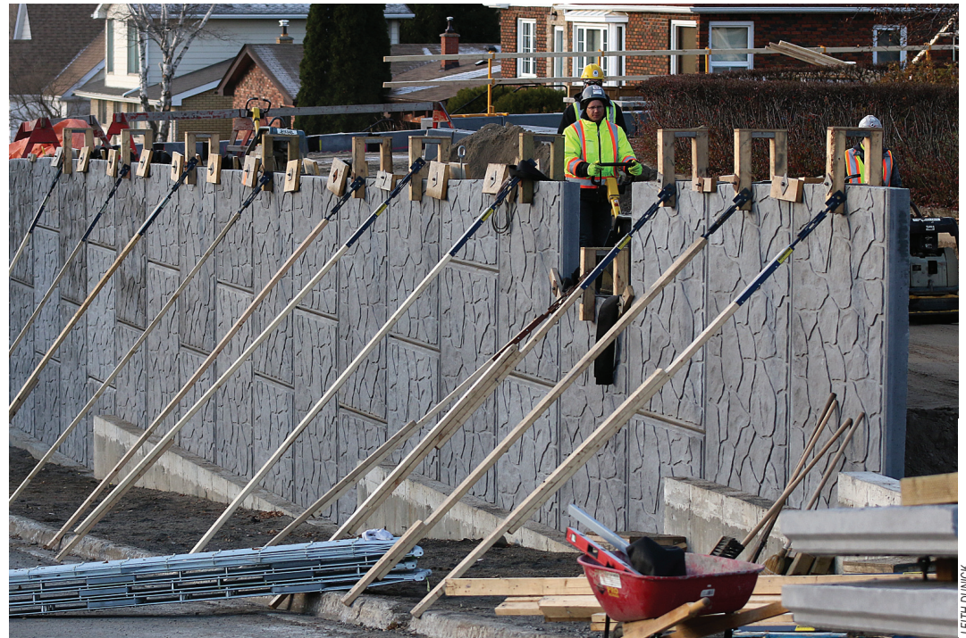
ALMOST FINISHED: Workers compact material behind a newly built, $2.1-million retaining wall on High Street.
